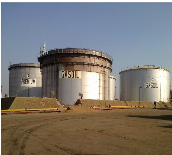
Above Ground Fuel Tanks
