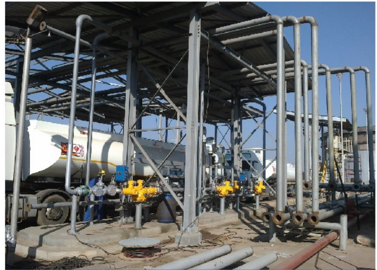
Gantry Works: Piping, Meters & Loading Arms
