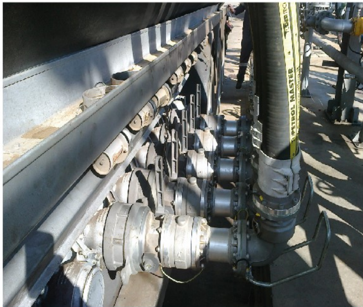
Truck Bottom Loading: Fuel Truck Bottom Loading
